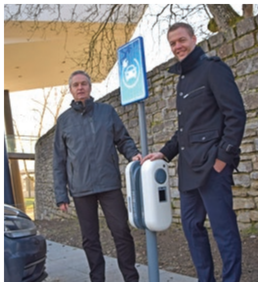
In 2020, Sto SE & Co. KGaA drew up plans for five further charging stations that will allow employees and guests to charge their electric vehicles from 2021.
